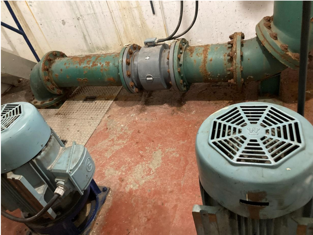
Motor Room – lift pump motors and combined pumps discharge line with flow meter
