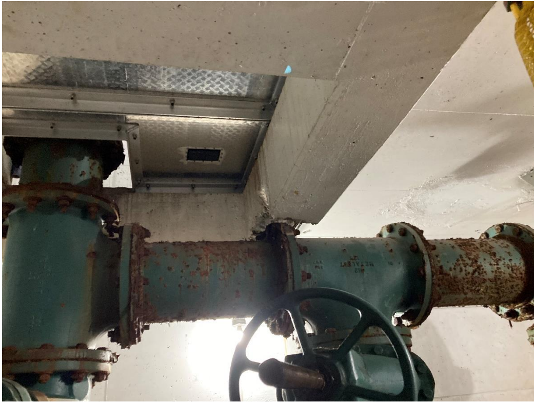
Pump Room – lift pump discharge header
