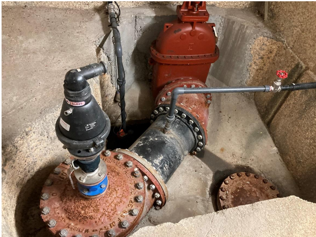
Comminutor Chamber - piping going to station wet well
