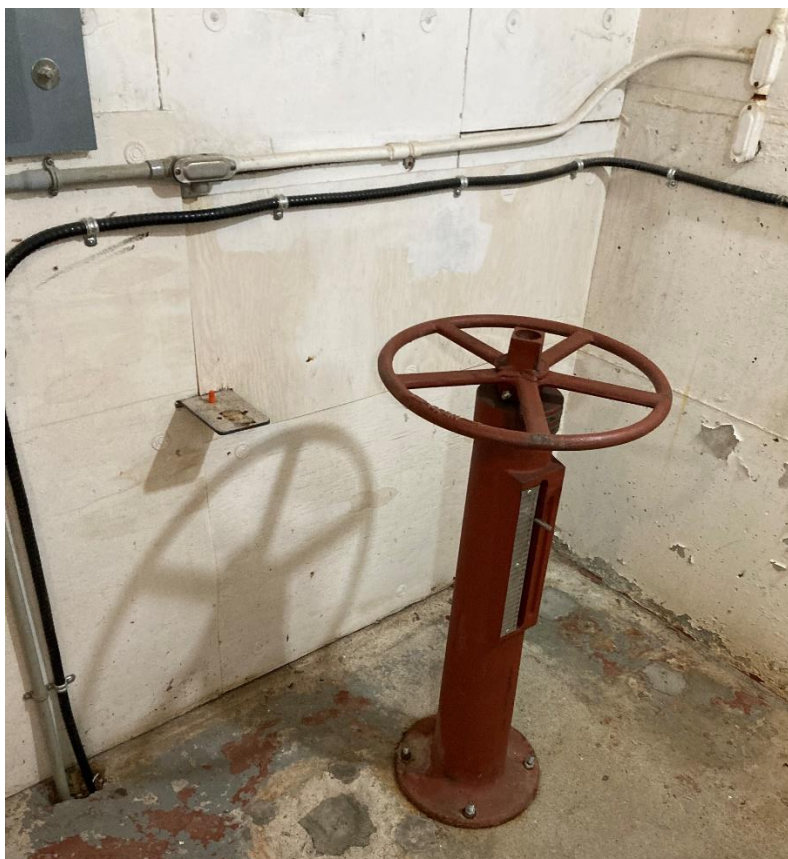
Lower Level – Valve Operator for Comminutor Chamber Gate Valve (right of CSO Panel)
