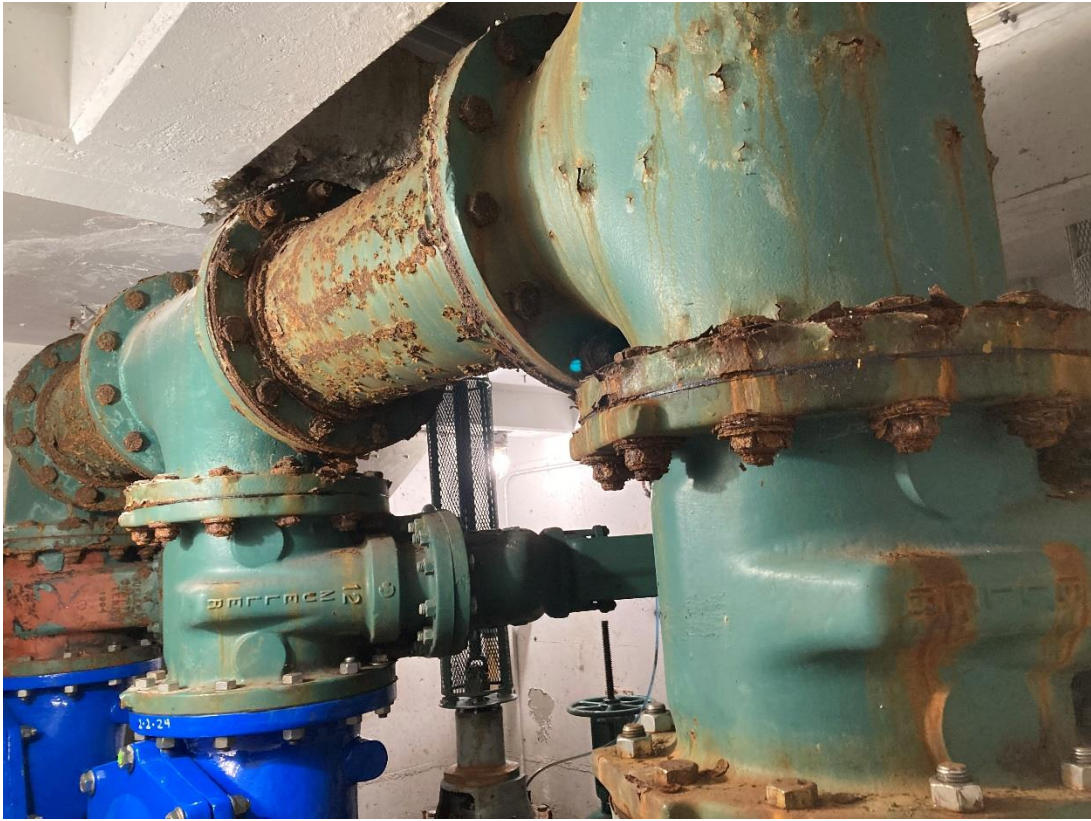
Pump Room – lift pump discharge header (lift pump 1 on left, lift pump 3 on right)
