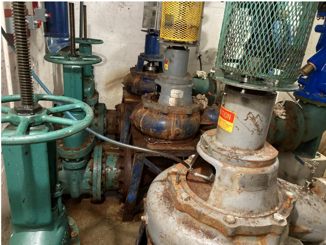
Pump Room – lift pumps and gate valves (lift pump 1 bottom, lift pump 3 top)
