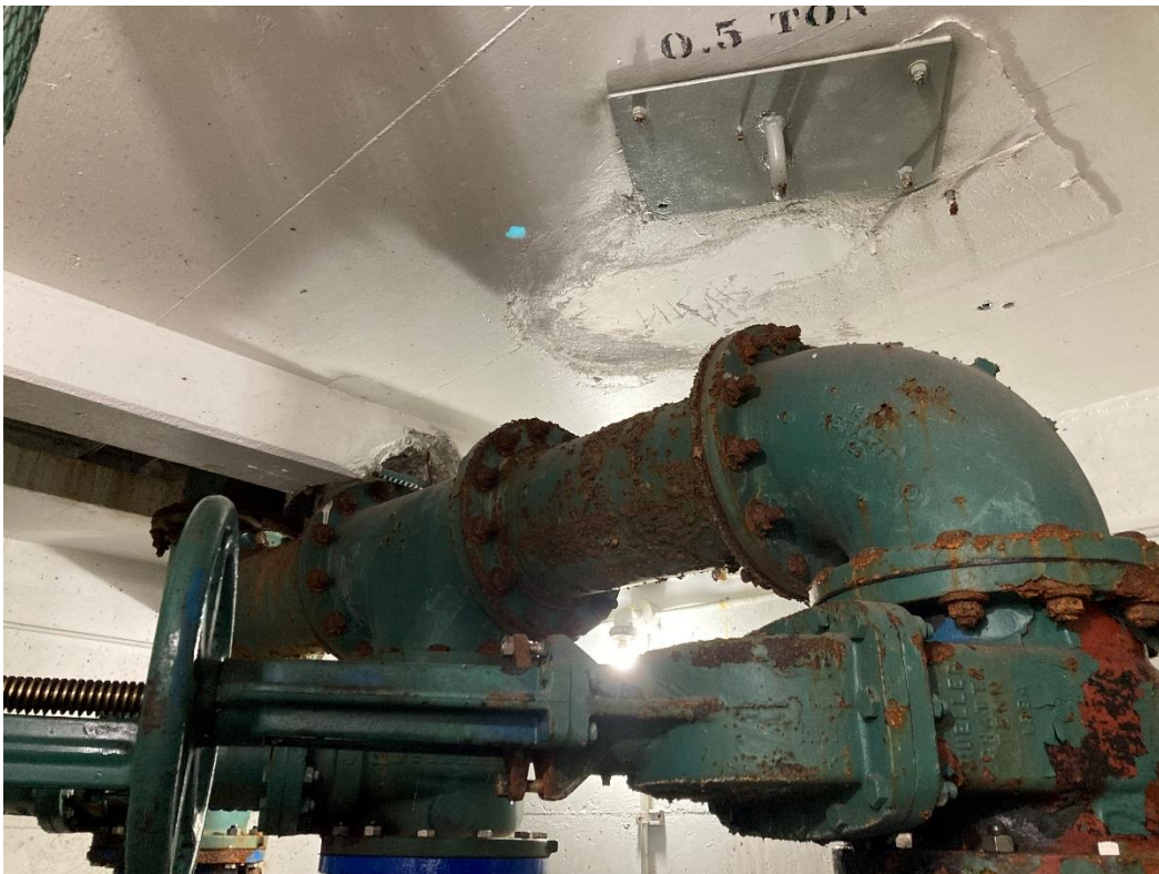
Pump Room – lift pump discharge header (lift pump 3 on left, lift pump 1 on right)
